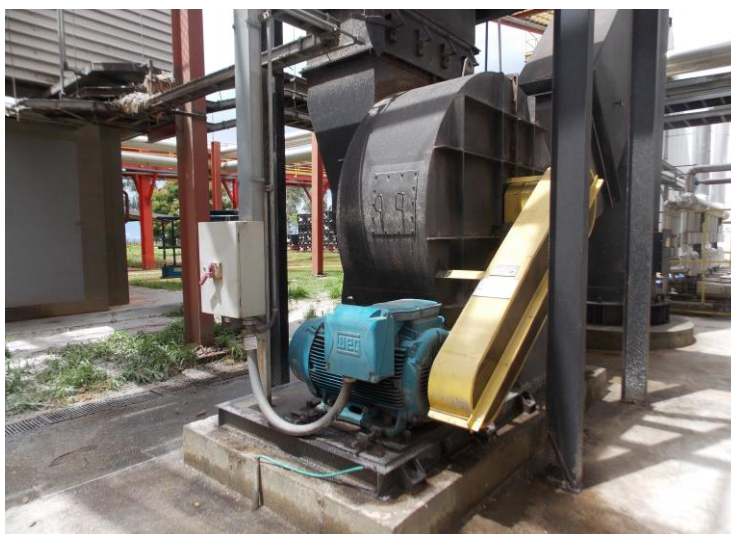
Figura 3-14 - Exaustor boiler BE-9075.
